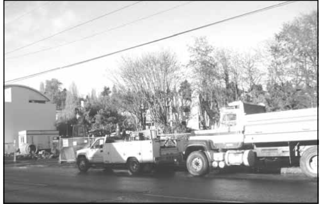
Madison Lofts construction site across the street from City Peoples Garden Store. Initially, the activity was cause of great concern as the holidays approached. MJR development has chosen to be a good neighbor!
