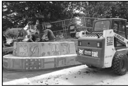
A Coyote Central installation in progress at the entrance to Powell Barnett Park
